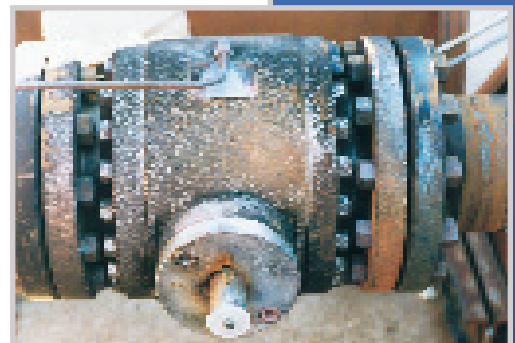
Successfully completed firesafe test.
